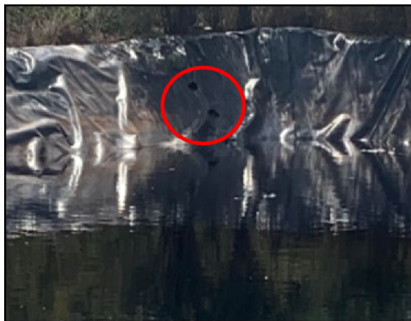
Figure 12. Damages to the geomembrane of the leachate treatment pond
