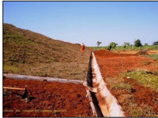
Figure 15. Drainage system that exists in the sanitary landfill of Cianorte by Albertin et al. (2011), PR.
